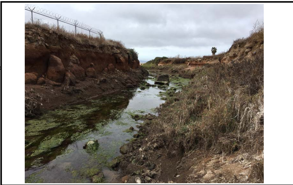
Photo 4. Photo taken from inside the eroding channel; just east of the proposed bridge span. Photo directed west toward San Diego Bay. Taken on 3/9/2018.
