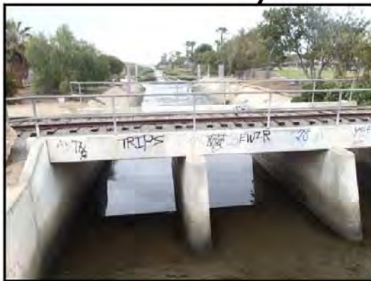
Looking west along the concrete lined portion of the J Street Channel.
