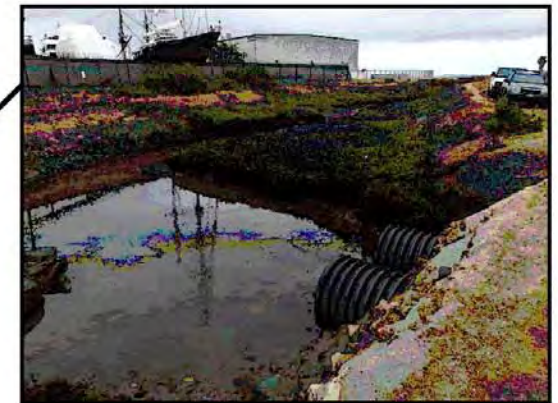
Twin 24-inch corrugated drains bring tidal waters to the F&G Street Marsh via a narrow entrance channel.
