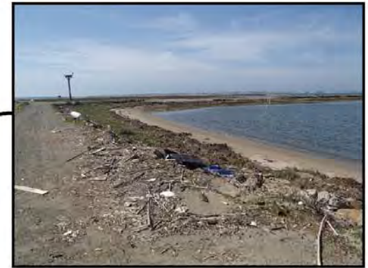
Looking west along the same portion of roadway. Presence of marine wrack is indicative of overtopping of the dike/ roadway during king tides.
