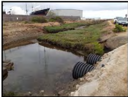
Twin 24-inch corrugated drains bring tidal waters to the F&G Street Marsh via a narrow entrance channel
