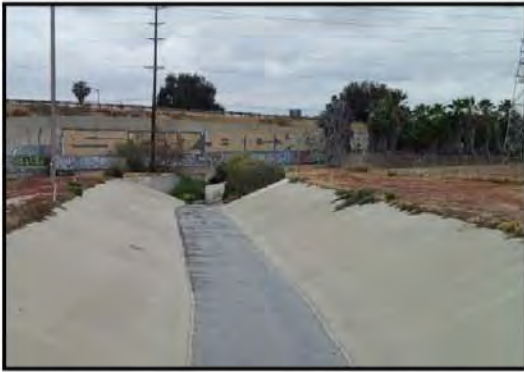
Looking east along concrete-lined Telegraph Creek before it crosses beneath Interstate 5 via a buried culvert.
