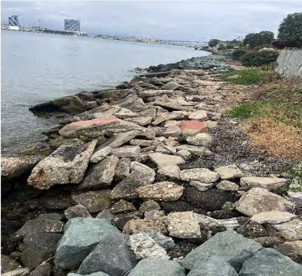
Exhibit 2-2. Construction Debris Fronting 409 First Street
