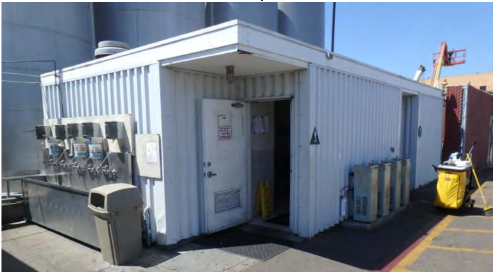
Existing pier 1 restroom to be demolished and incorporated into new admin complex
